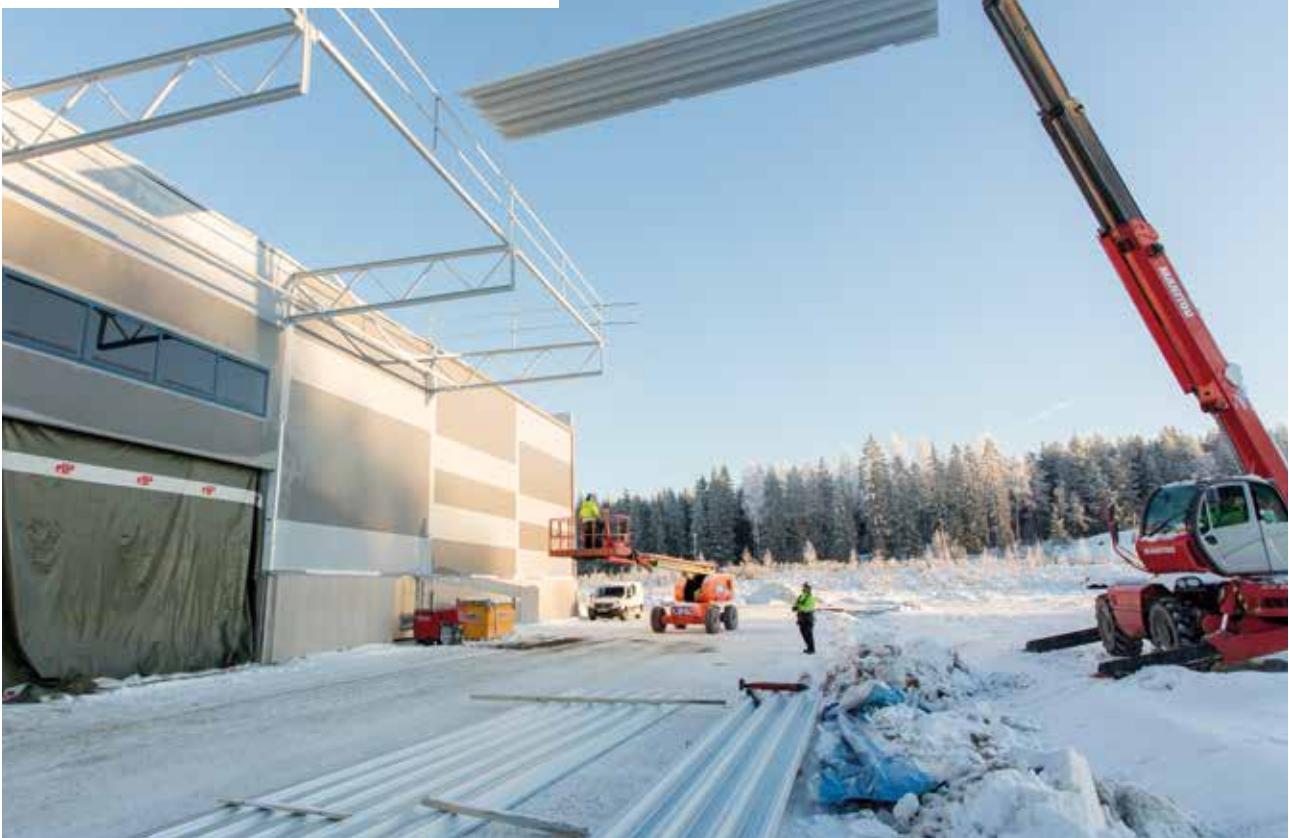
On the Sothönan 3 property in Katrineholm, Catena began construction of a 10,000 square-metre terminal to handle heavier industrial products that impose specific demands on handling capabilities, but less on temperature.
